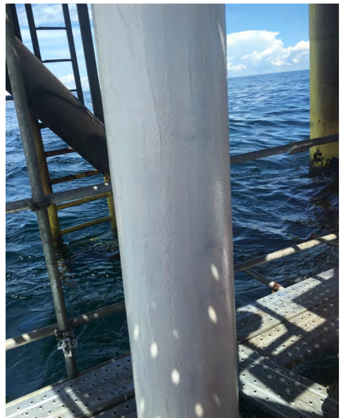
Figure 4. Three crude oil risers located in Southeast Asia were experiencing external corrosion and were repaired by utilising the SplashBond™ primer.
