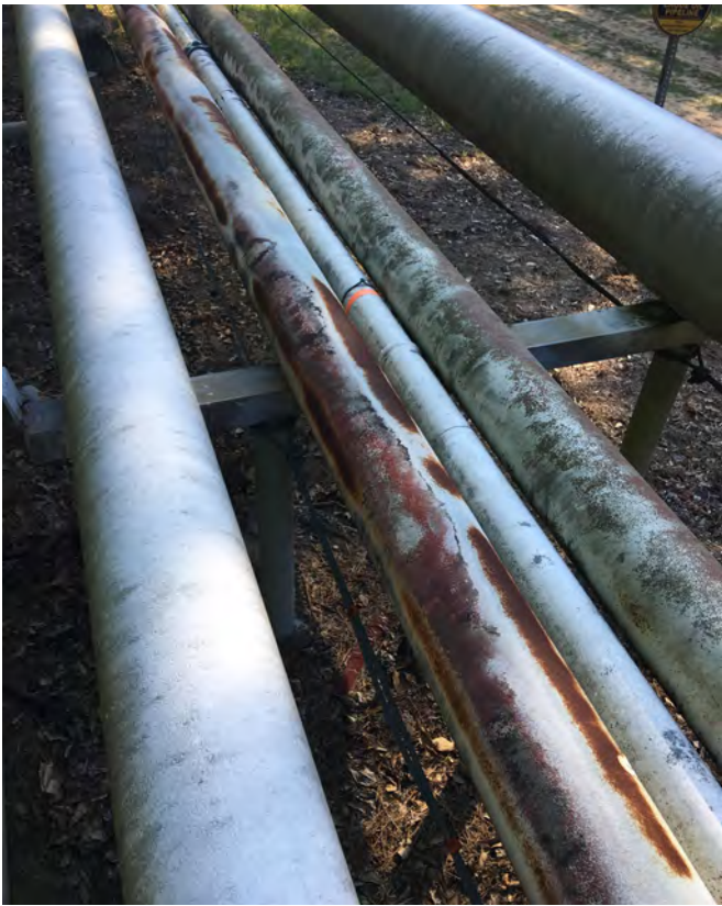
Figure 1. It is common for pipelines to experience abrasion and corrosion at support and hanger locations.
