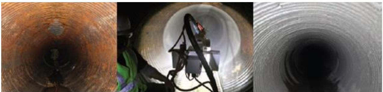
Figure 2: From left to right (a) Leaking storm water culvert (b) Centrifugal application of GeoSpray™ (c) Completed Repair 11
