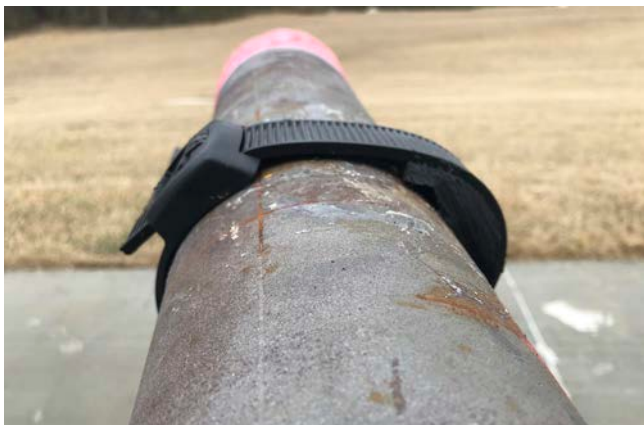
Figure 3. A completed Leak Stopper installation has a low profile that allows it to be overwrapped with a composite for a long-lasting repair.
