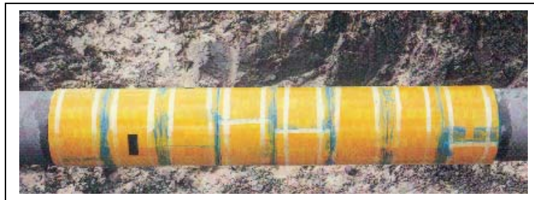
Figure 1. Multiple Clock Spring® Units
